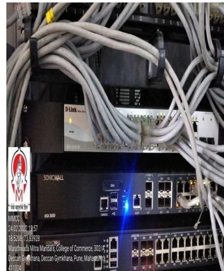
Fire Wall ( Computer Laboratory)
